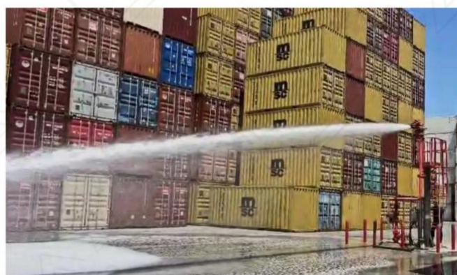
Foam Monitor of Port Project in Thailand
