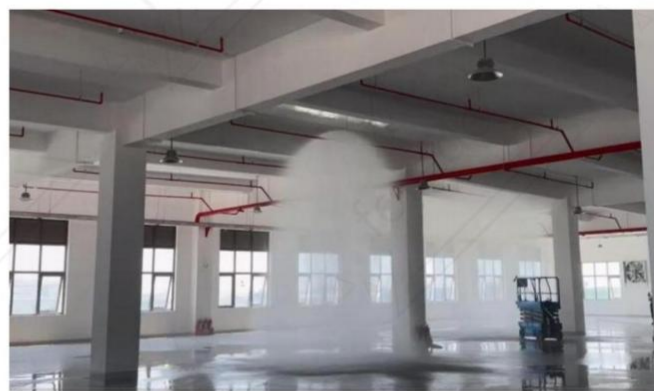
Fire Sprinklers in Myanmar
